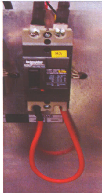
Picture 2 : D.C Terminals Short Circuited
