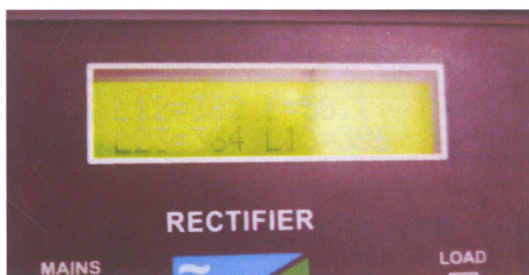
Picture 3 : Incoming Connected to the AC
